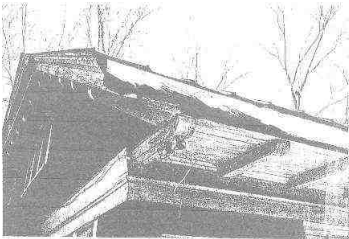
Figure 4k. Rotten fascia and soffit of Carriage House from leaking roof and squirrels.
